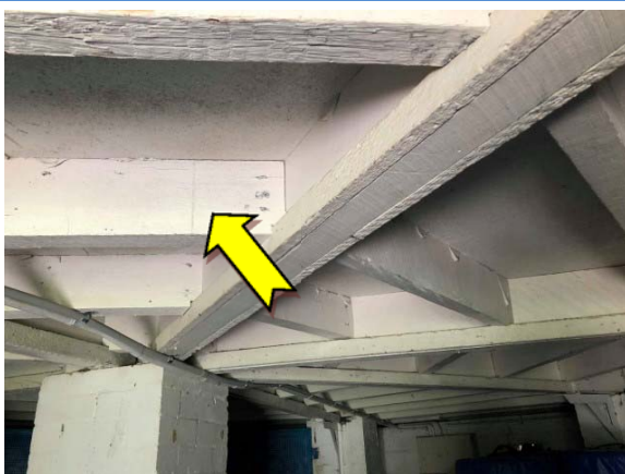
Photo 5. Interior, subfloor, walls, ceiling and timber slats – suspected lead-containing white upper paint systems.
