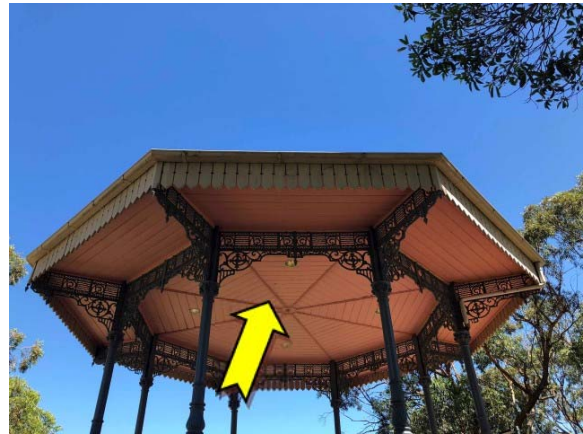
Photo 4. Exterior, throughout, ceiling – suspected lead-containing pink upper paint systems.
