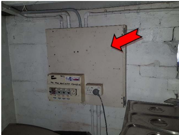
Photo 3. Interior, subfloor, electrical backing board – suspected asbestos-containing bituminous backing board.
